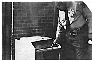
A centrally located computer terminal permits a security guard to quickly obtain a status report on conditions within the building.
